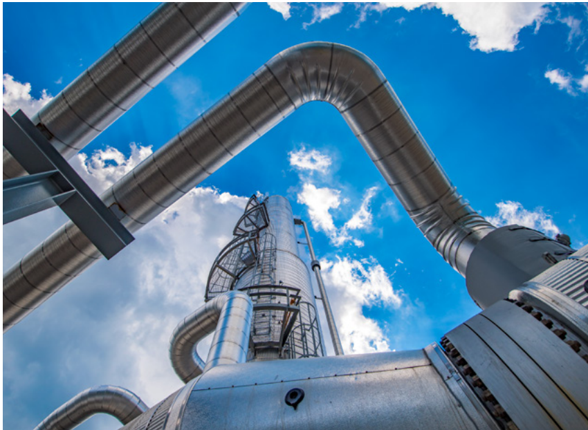
On the cover: Sherwood natural gas processing plant in Doddridge County, West Virginia – the largest gas processing plant in the U.S.
